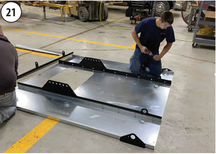
Assemble the tailgate latch by bolting (1) trip arm mount to each side of the tailgate assembly with (2) 5/16"-18 x 1" flange screws & 5/16"-18 locknuts.
